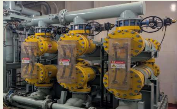
BWTS installed on SCI VLCC DESH VIRAT
