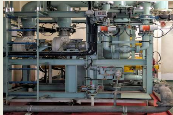
BWTS installed on SCI VLCC DESH VIRAT
